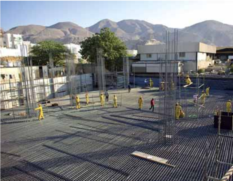
The sector has recently witnessed a push towards cleaner, more efficient building methods
